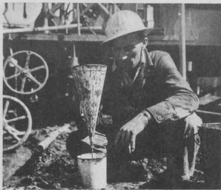
8 As the drill bits tore at the underground rock, specially prepared mud was pumped down the pipe to be returned to the top carrying up rock cuttings. Here the mud is being tested
